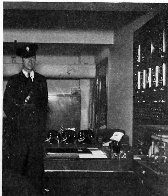
Police-booth panel board controlling microphones and amplifiers in large group of safe-deposit vaults. Presence of anyone in any vault can be detected during regular patrol sequence. For test purposes, gong automatically sounds in each vault to make sure amplifier circuits are working
